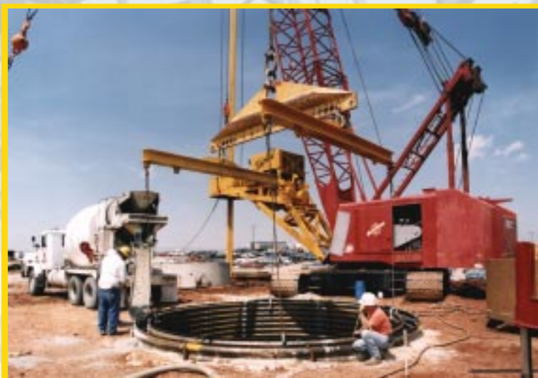
CEMENTING OF THE 17.5-FOOT DIAMETER CASING TO THE TOP OF THE LIMESTONE LAYER.
