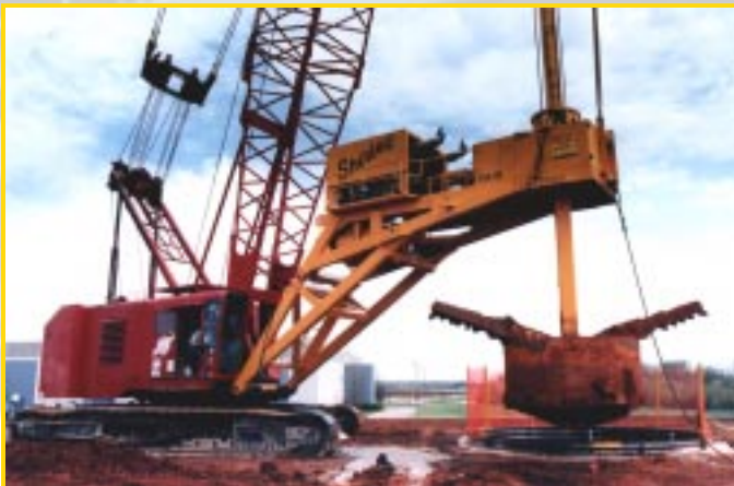
DRILLING CLAY, 19.5-FOOT DIAMETER, TO 50 FEET DEEP TO TOP OF LIME STONE LAYER.
