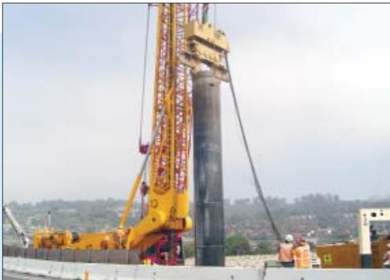
Installing the 60" diameter steel casing with an "APE" King Kong dual-clamp vibratory hammer, Abutment 1.
