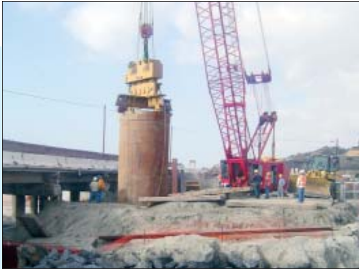
Installing the 111" diameter steel casing with a King Kong quad-clamp vibratory hammer, Pier 3.
